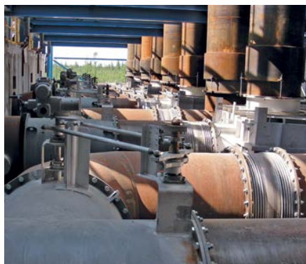
US-types installed in a flue gas system.
