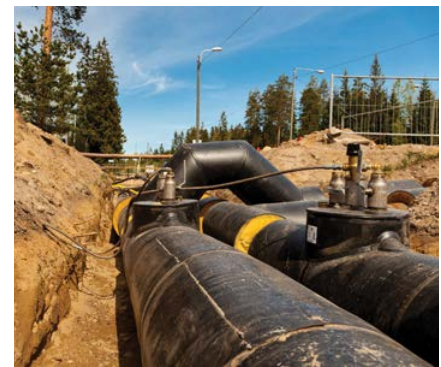
District heating pipeline.
