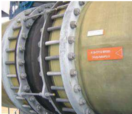
GRP Cooling Water Piping.
